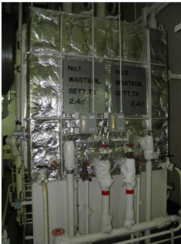
The Waste Oil Settling Tanks
