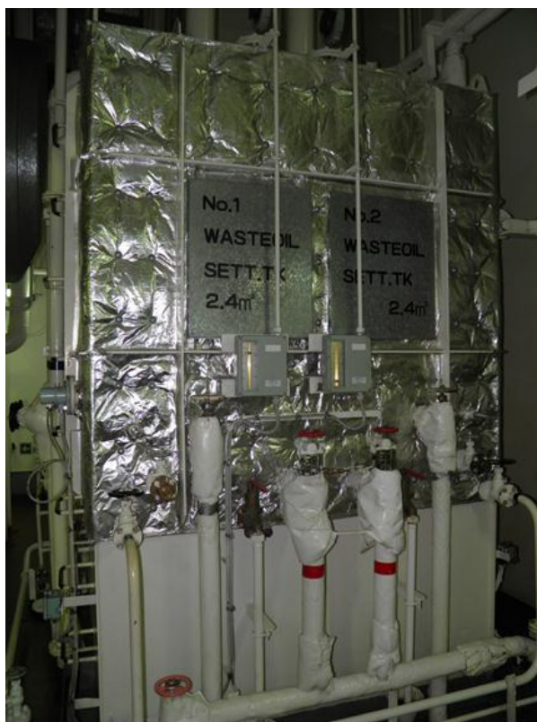
The Waste Oil Settling Tanks
